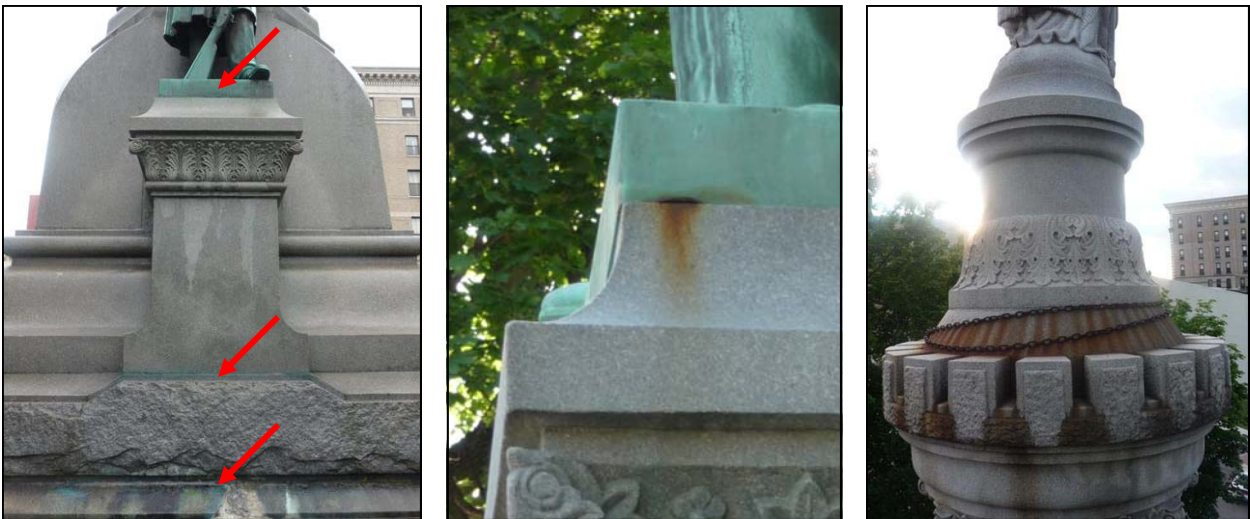
Figures 21-23. Examples of copper staining (left), mild and significant rust staining (center and right, respectively) on the monument.
