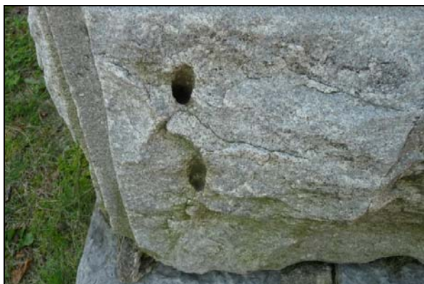
Figure 8. Example of voids caused during original construction.
