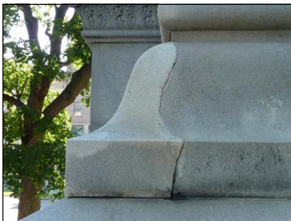
Figure 10. Point-loading has caused one corner of the cyma level to separate at a fracture line.
