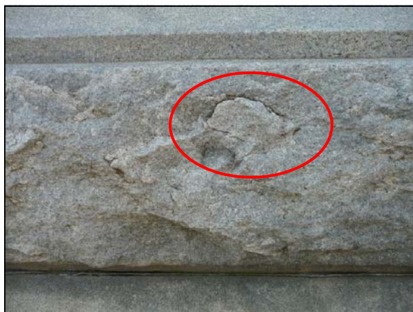
Figure 9. Minor incipient spalls on the face of the base stones are due to the original technique used to create the pitch-faced finish of the stone.
