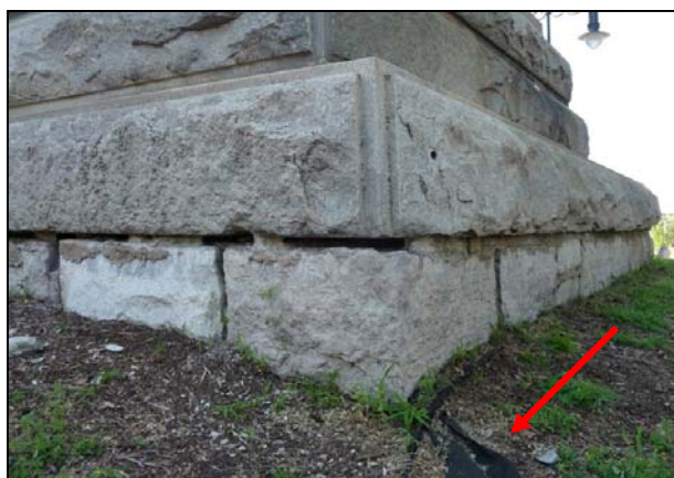
Figure 16. General condition of the foundation (lower course). Also note the emergence of the landscape fabric.
